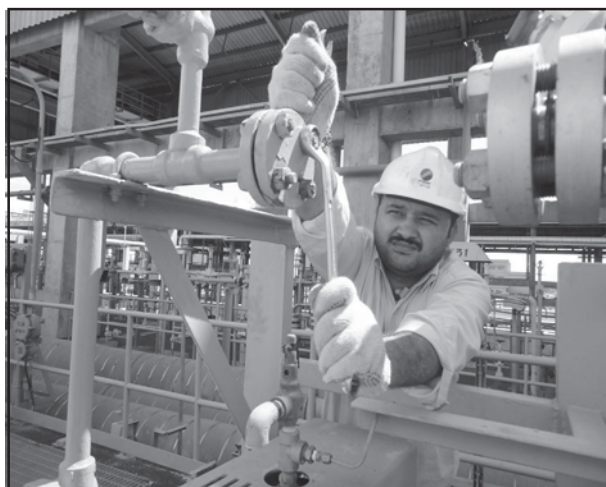
Employee working at Dahej LNG Terminal
