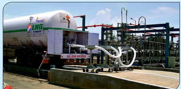
Truck loading facility at Dahej.
