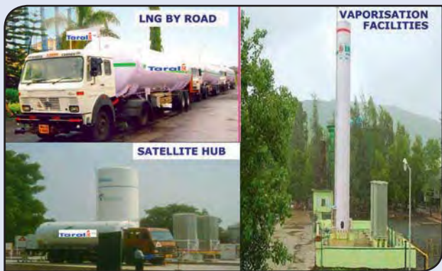
Facilities for Supply of LNG by Road
