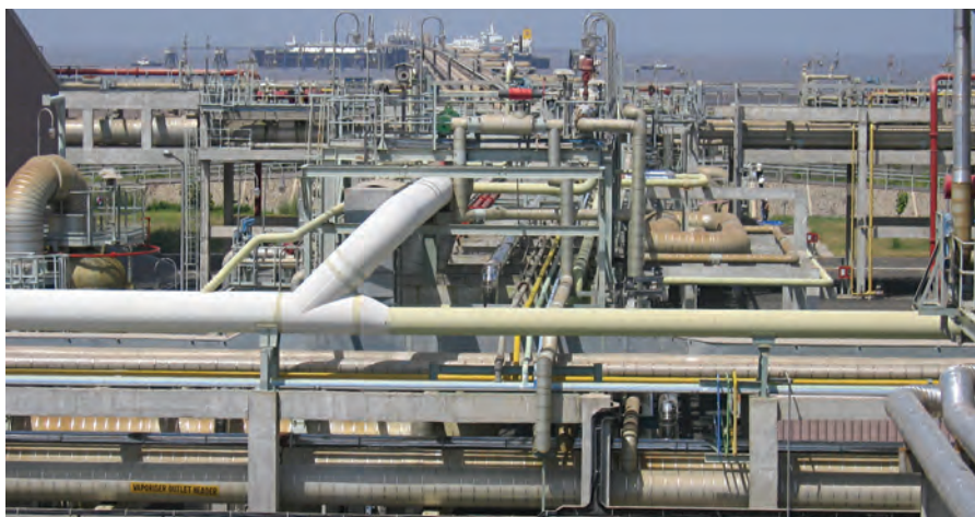
Dhahej Terminal- Pipeline view
