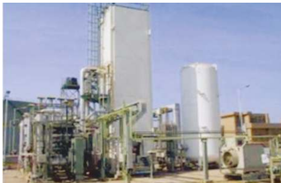
Liquid Nitrogen Plant
