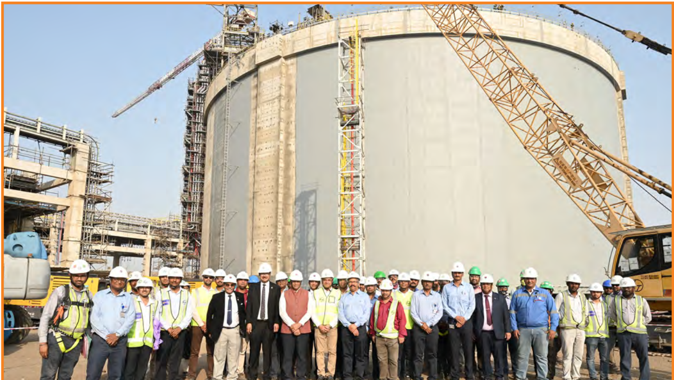
Shri Pankaj Jain, Chairman, PLL at the tank inauguration at Dahej LNG Terminal
