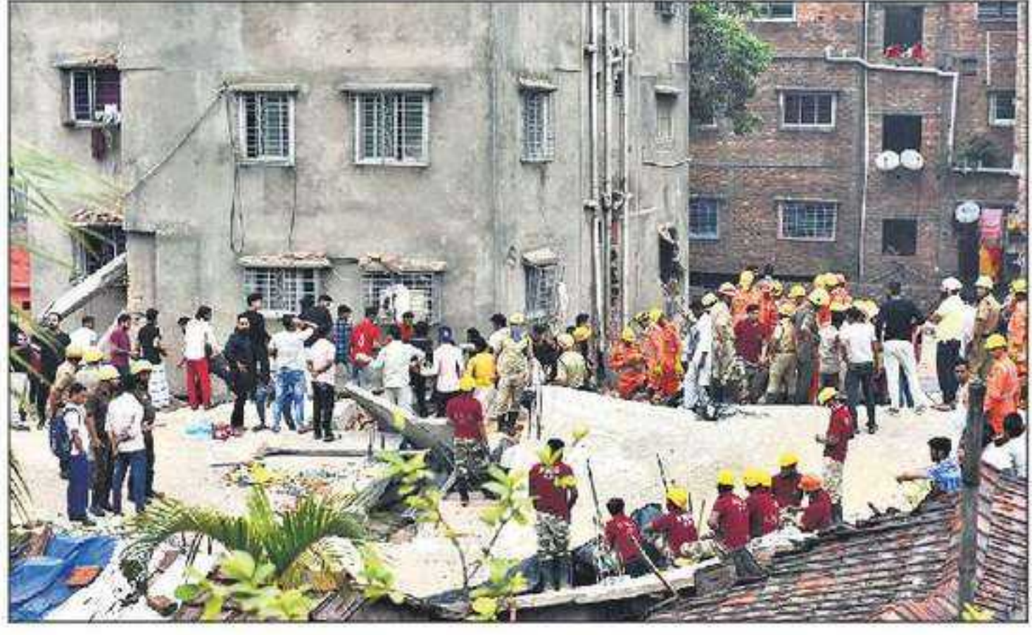
Rescue operation underway after an under-construction building collapsed at Garden Reach area in Kolkata on Monday. HT PHOTO
