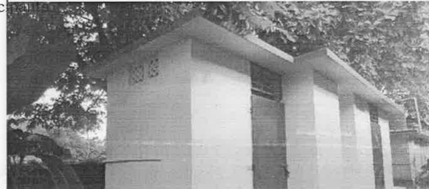
21 Toilets constructed in the schools by Wockhart Foundation Toilets in the year 2015-2016. Out of the two work orders issued of amount Rs 13.38 Lakhs dated 19.03.2016 and Rs 6.40 Lakhs dated 04.08.2016 and amount 85 % of the total amount and 50 % has been released to the party M/S Wockhardt
