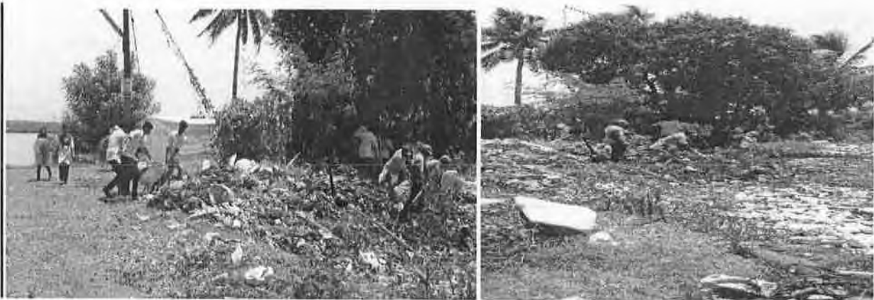
Habitat improvement work at Cherrai on 27.8.16 to 30.8.16 in association with NSS members of Gov. Polytechnique, Kalamassery and Kudumbasree unit Cherrai
